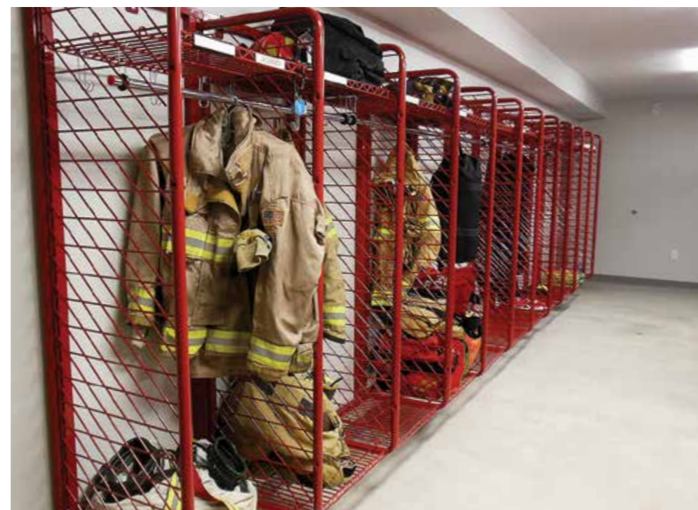
A special ventilation system in the personal protective equipment turnout room allows fumes and contaminants to vent outside the building, protecting the firefighters from harmful carcinogens.
